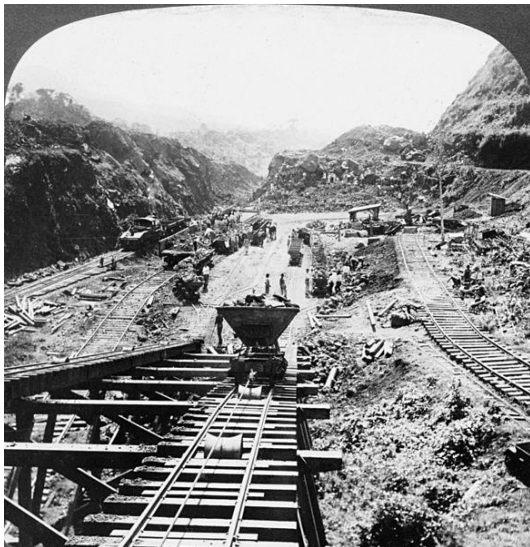
H.C. White Co. - Where the work is being pushed with greatest energy - the famous Culebra Cut, Panama Canal, April 8, 1907 Library of Congress, Prints and Photographs Division, Washington, DC
